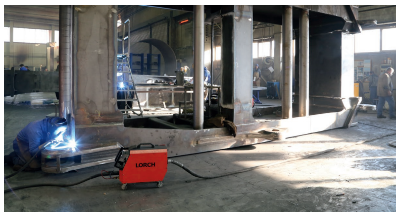
A total of 42 welding units of the Lorch S-SpeedPulse-XT series ensure excellent weld seams at ADK.
